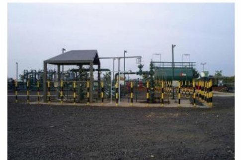
SALTFLEETBY B - GAS PRODUCTION EQUIPMENT
